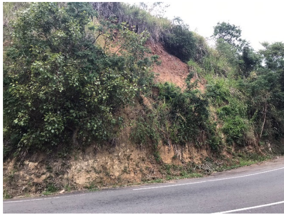
Unstable slope area
