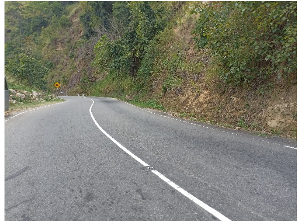
Unstable slope and the Ella-Wellawaya (A23) road
